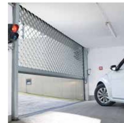
TG-A roller grille in an underground garage
