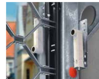
8 Photocells (roller grilles) The roller grille gate has additional photocells around the lintel to prevent personal injury.
